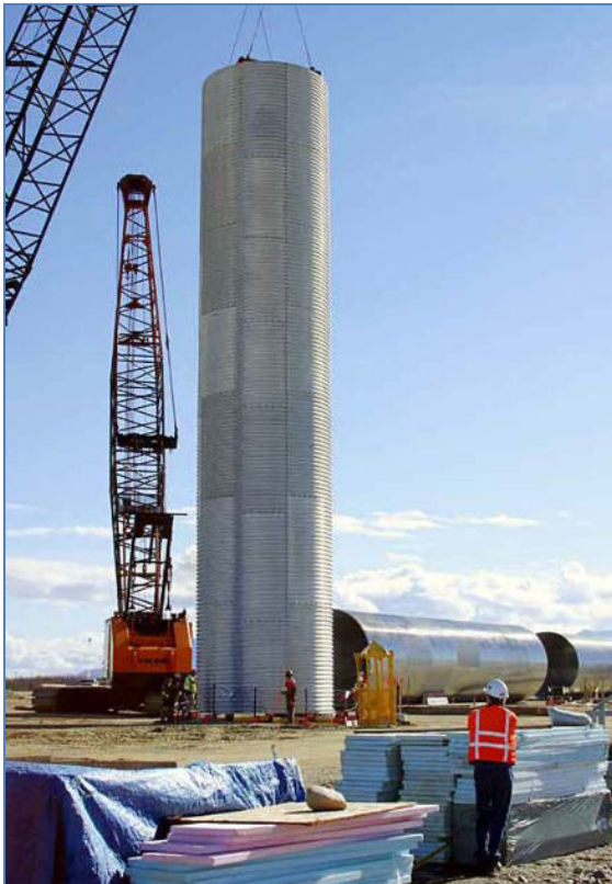
Figure 107: A silo liner being lifted into place for installation into a missile silo at a launch complex under construction. (The Boeing Company)
